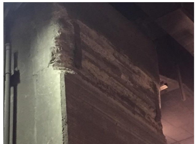
Figure 9. Column in intersection of X axis and 7 axis in Level +19.00. Significant change of cross section is observed (Source:Own)
