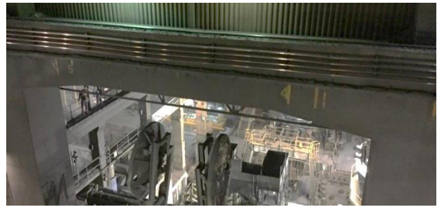
Figure 12. Rail beam between axles C / 6 and C / 7 (Source:Own)
