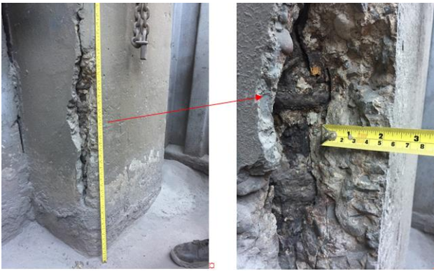
Figure 10. Column damaged on axis C / 3 Level 0.00. (Source:Own)
