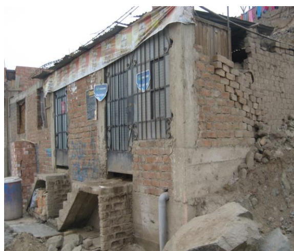
Figure 1. Non engineering confined masonry dwelling.
