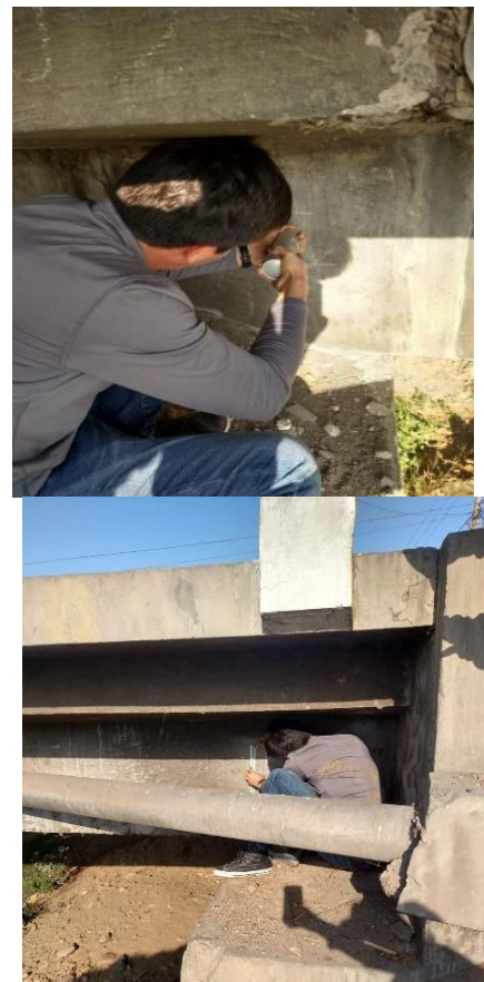
Fig. 6. Non-destructive in-situ sclerometer compression test of Points 1 and 2 of the main girder of the Moche bridge.
